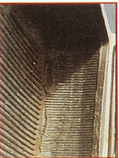
Cracked drop-in liner
